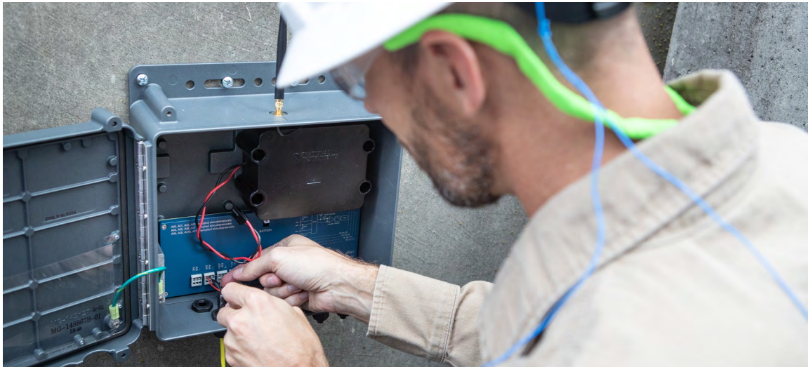
Figure 2. An engineer installs a wireless device and accelerometers to monitor three cooling towers.
